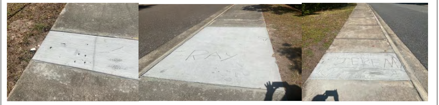
New Sidewalk that was Damaged
